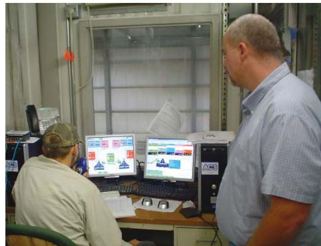
Conewago Batching Operator Mike Unger, seated, and Plant Manager Kevin Gladis use the PCS Computer Control System from ACS to fine-tune planned batch runs for the day. The graphical user interface shows the operator exactly what is taking place or planned at any point in time. Up to 1,000 recipes can be stored and recalled at the touch of a button.
