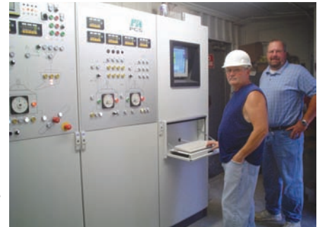
Under control - Northern Concrete Pipe GM Scott Boughner, left, and President Bill Washabaugh Jr. found the right recipe for total plant control in the ACS Programmable Control System (PCS). Improved accuracy, consistency, and reliability are resulting in better quality and happy customers.
