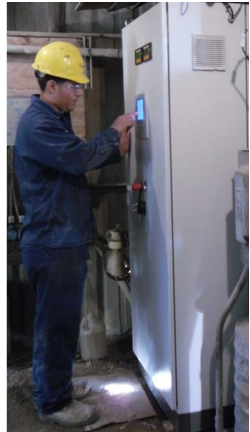
The self-contained ACS Smart-Touch Control System can be located anywhere on the plant floor. Here, operator Javier Sanchez sets up for the day's pipe run at Hanson's Helmers Street plant using the Smart-Touch touch screen panel. The Helmers Street control upgrade, which included controls for two separate production lines, was completed over a weekend.
