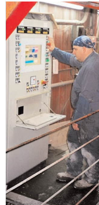
A&R QC manager Chris Ferranti glances at the production screen of the new SmartMix panel. He was pleasantly surprised when the new ACS components increased the batching speed of the plant. He now has the flexibility to switch easily between manual and automatic production. The SmartMix system produces and records all the data critical for Chris's daily QC reports and functions.
