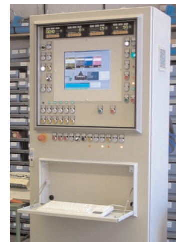
The ACS SmartMix control system goes through final production simulation testing and a final check before it is shipped to Granite. Pre-configuration helps minimize installation downtime. The all-in-one display delivers a comprehensive view of all plant operations.
